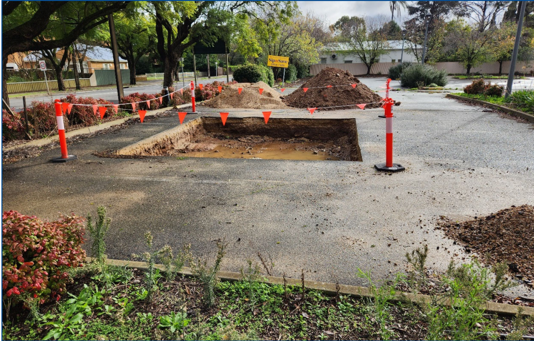
Photograph 5: View of the A-BH01 soil excavation as part of AME's soil validation works. The resultant soils have been temporarily stockpiled on-site pending future off-site disposal.
